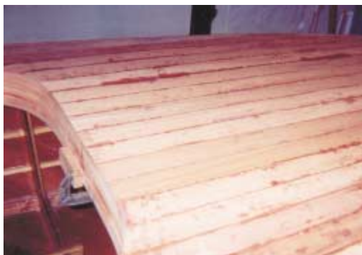
The final planking layer was 1/8" African mahogany. The total project consumed some 60,000 staples of which 55,000 were pulled after the epoxy was set.
