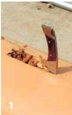
Figure 2—Once the mast was split open, the full extent of the rotted area was revealed.
