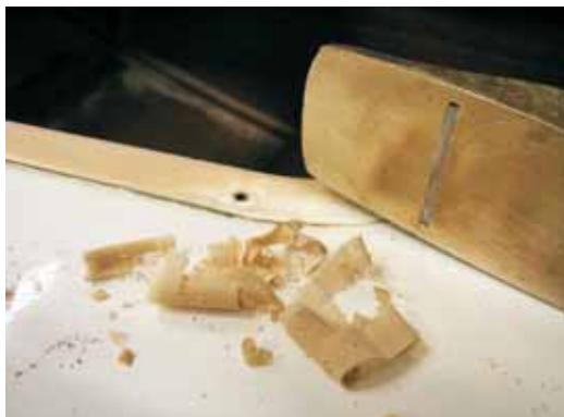
Photo 2—One side of the new larger hatch was in the same location as a side of the old hatch. The low-density epoxy/410 Microlight mixture along that edge was easily removed with a low-angle block plane.
