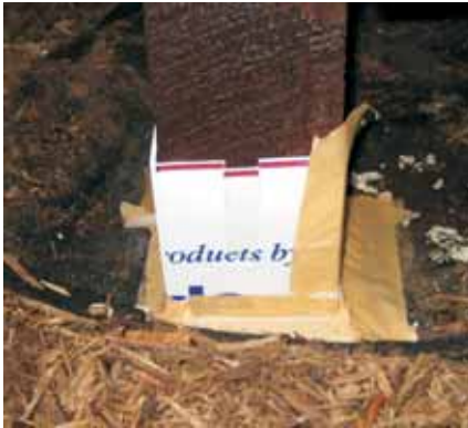
After treating the posts with wood preservative, Blackmon used plastic sign material to make forms around the base of the posts.
