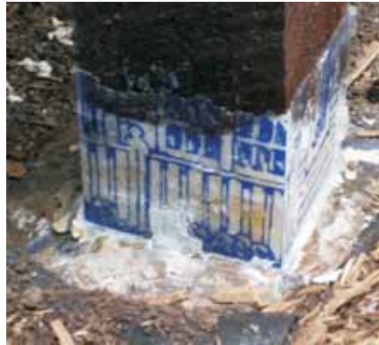
The forms were removed from the cured epoxy revealing the ink that transferred from the inside of the form to the epoxy.
