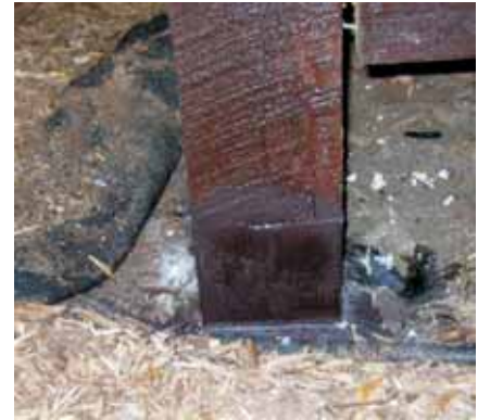
Blackmon finished the repair with a coat of dull brown paint to camouflage the epoxy base.
