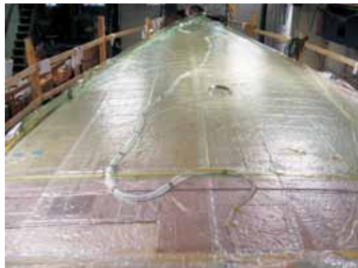
Two layers of 1/4" plywood are vacuum bagged over cedar planking. Note the staggered joints in the plies.
