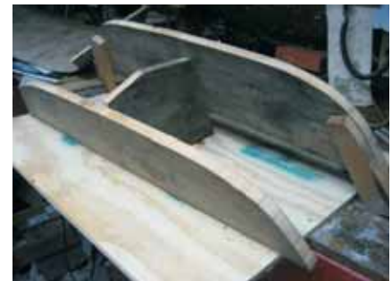
The foam with reinforcement on only one side was then placed over this male form and glass was added to the outside surface.
