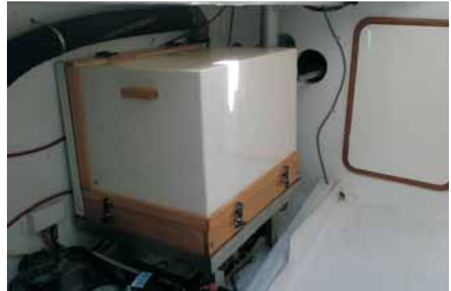
The generator with the soundproof enclosure in place.
