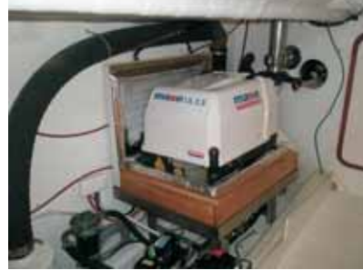
The generator installed on its soundproofed base.
